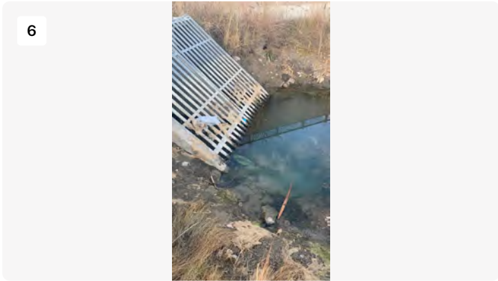
as part of the repair work we propose to lift of these gates and clean out this inlet.
