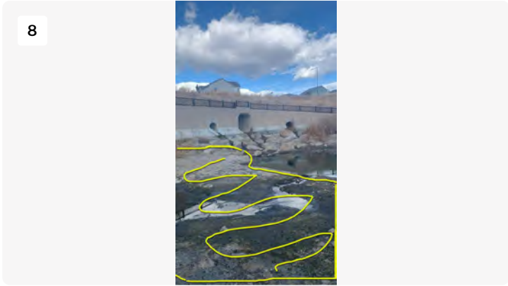
The plans show a spillway full of large boulders embedded in concrete. some of these boulders are covered. we need to uncover them and remove excess sediment here.
