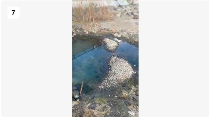
Another angle. all of this rock and sediment needs to come out. at Yucca.
